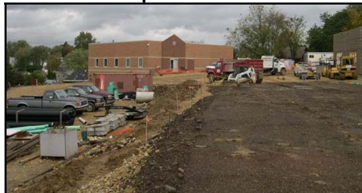
View of the Facility Building, with construction of the Chlapaty Center underway at the University of Dubuque.
