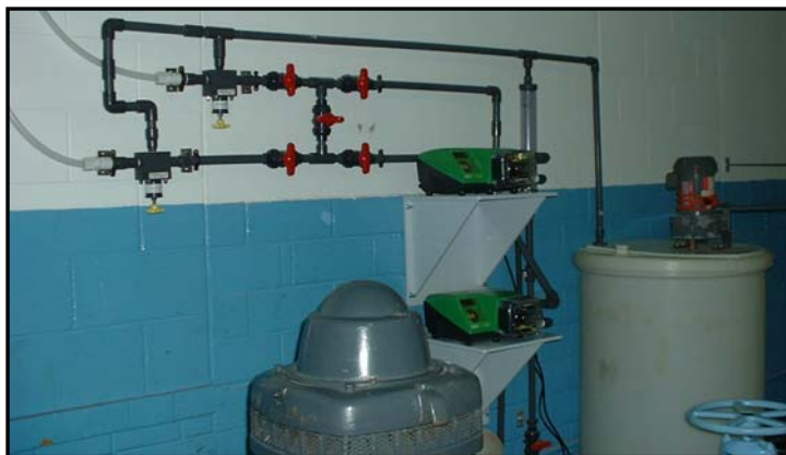
New chemical equipment at Forest City Water Treatment Facility.
