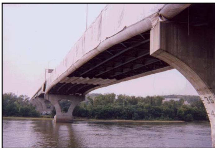
The contractor utilized a containment system and filtration systems to safely remove and dispose of lead paint dust and blast media.
