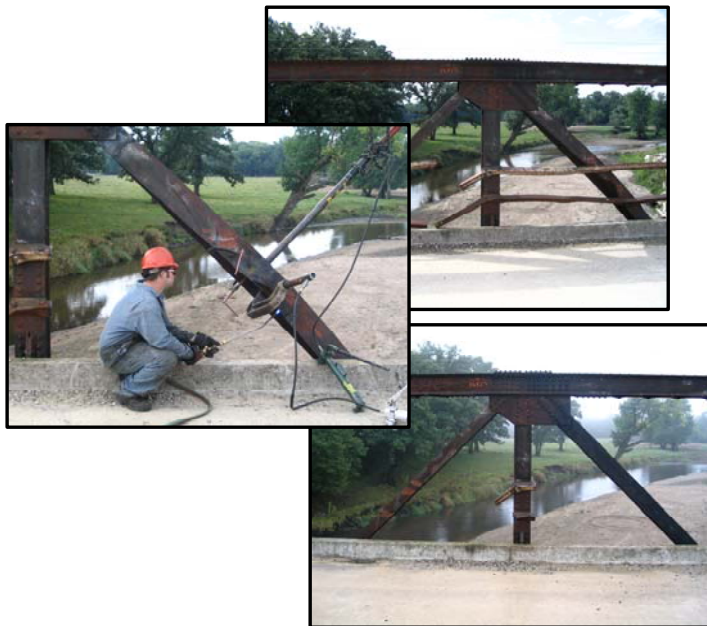
Heat-straightening is a quick and economical method used to straighten structural steel members.
