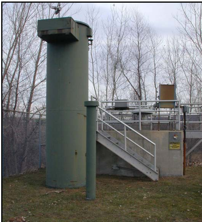
Existing entrance to dog track lift station.
