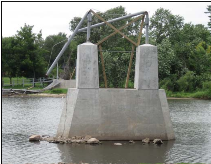
Devastation to the Charles City, Iowa Pedestrian Bridge.
