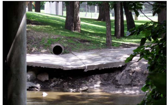
Undermining of the sidewalk at the south end of the bridge location at 1 st Street at Willow Creek Bridge in Mason City, Iowa.
