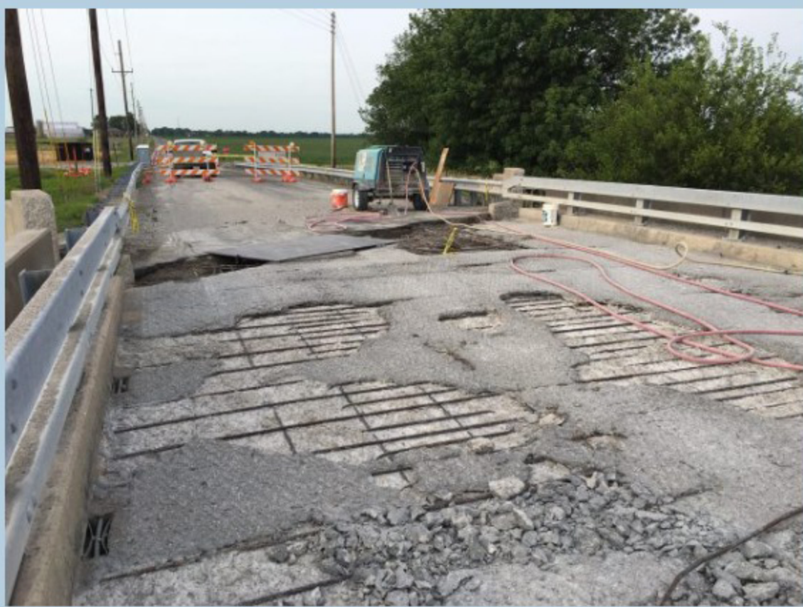
Damaged Deck After Hydro-Scarification
